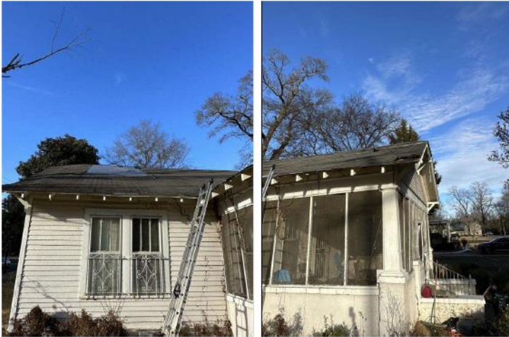
1.0 The roof covering is old, and the life of covering has expired. The covering does need to be replaced.
